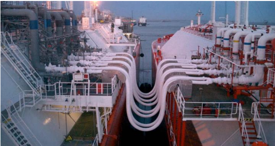
Figure 2: LNG transfer between LNG carrier and FSU via flexible cryogenic hoses.
