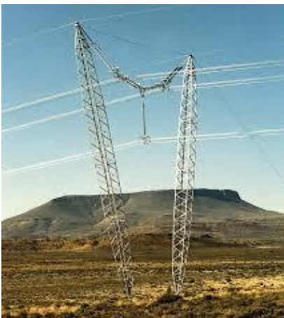
Figure 57: Typical transmission powerline support structure/ tower.
