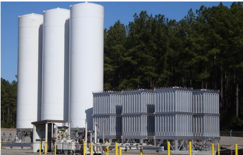
Figure 8: Typical vertical LNG cryogenic bulk storage tanks. A single 300m 3 storage tank typically stores 145 tonnes of LNG.
