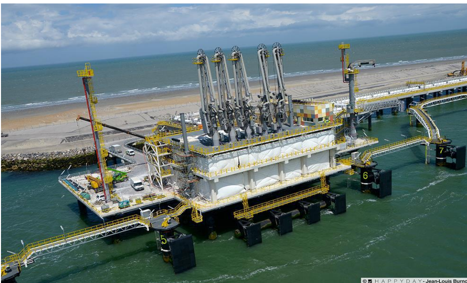
Figure 4: LNG vessel docking/ mooring station complete with LNG cryogenic unloading arms located on the LNG Terminal.
